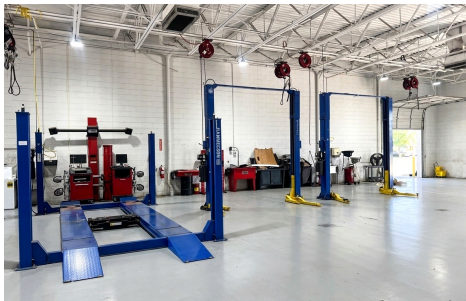
Open service floor — two-post lifts, alignment rack & overhead hose reels in place
