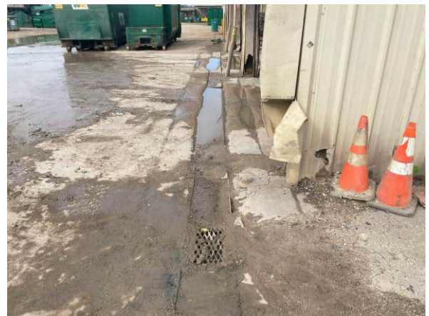
Photo 28 View of an on-site trench drain (Tract 2)
