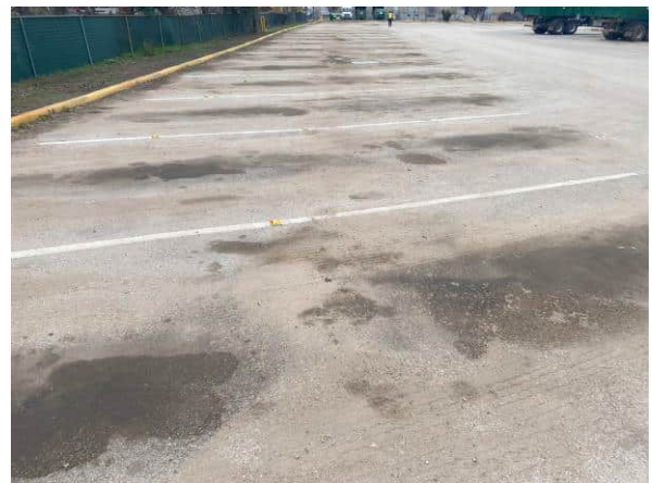
Photo 22 Typical view of de minimis staining in the garbage truck parking area (Tract 2)
