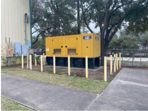
Photo 31 View of an on-site emergency generator (Tract 2)
