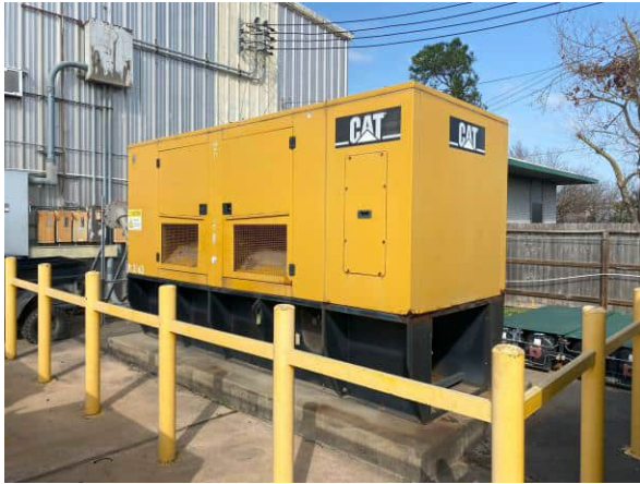
Photo 13 View of an on-site emergency generator (Tract 1)
