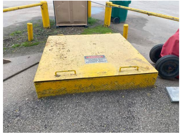
Photo 20 View of an apparent sump associated with the on-site ASTs (Tract 2)
