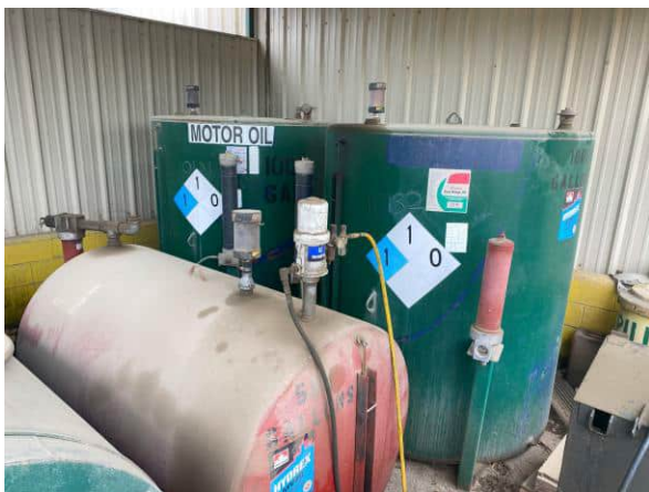
Photo 23 Typical view of the on-site oil ASTs (Tract 2)
