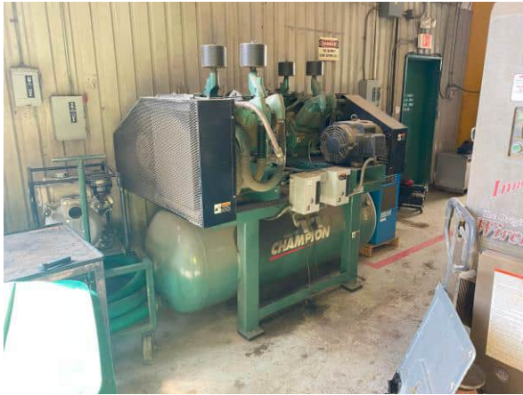
Photo 7 View of an on-site air compressor (Tract 1)
