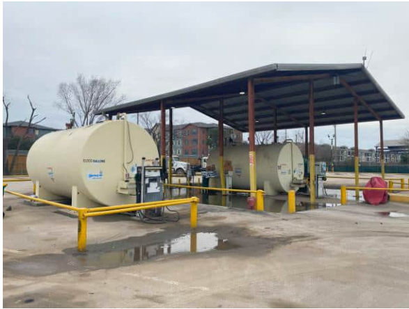
Photo 19 View of the on-site diesel ASTs (Tract 2)
