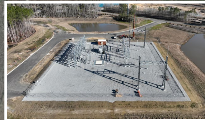
On-Site Palmetto Electric Substation
