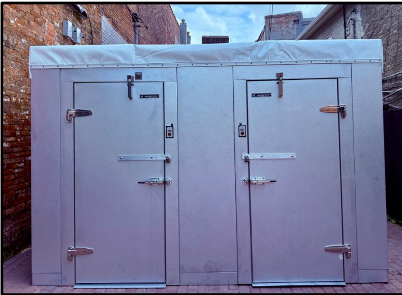
PICTURE 2: 12X12 WALK IN REFRIGERATION & FREEZER
