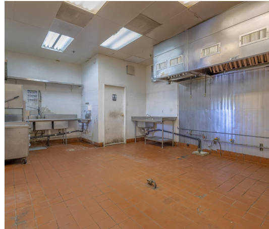
KITCHEN - TYPE I HOOD IN PLACE
