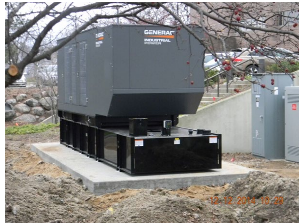
BUILDING WIDE BACK-UP GENERATOR
