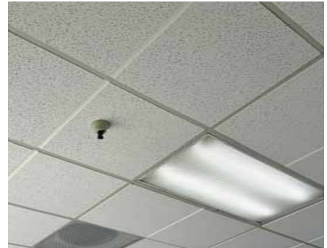
3093 McKee Road - Fire Sprinklered
