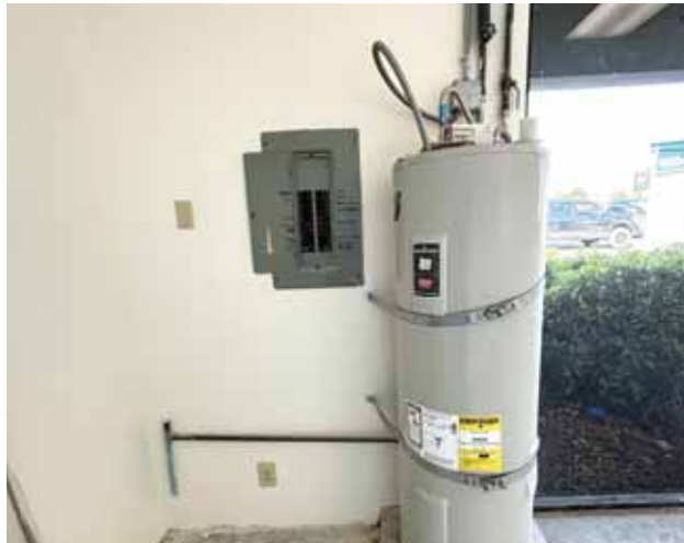
Electrical Panel & 40-Gallon Electric Hot Water Heater
