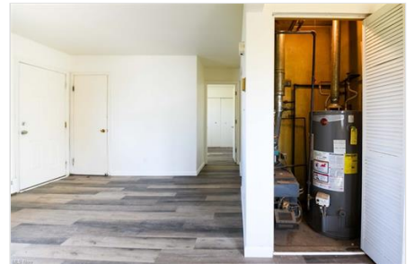
Utility room with water heater
