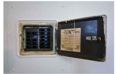
View of utility room
