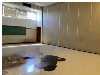
Leak f roof
