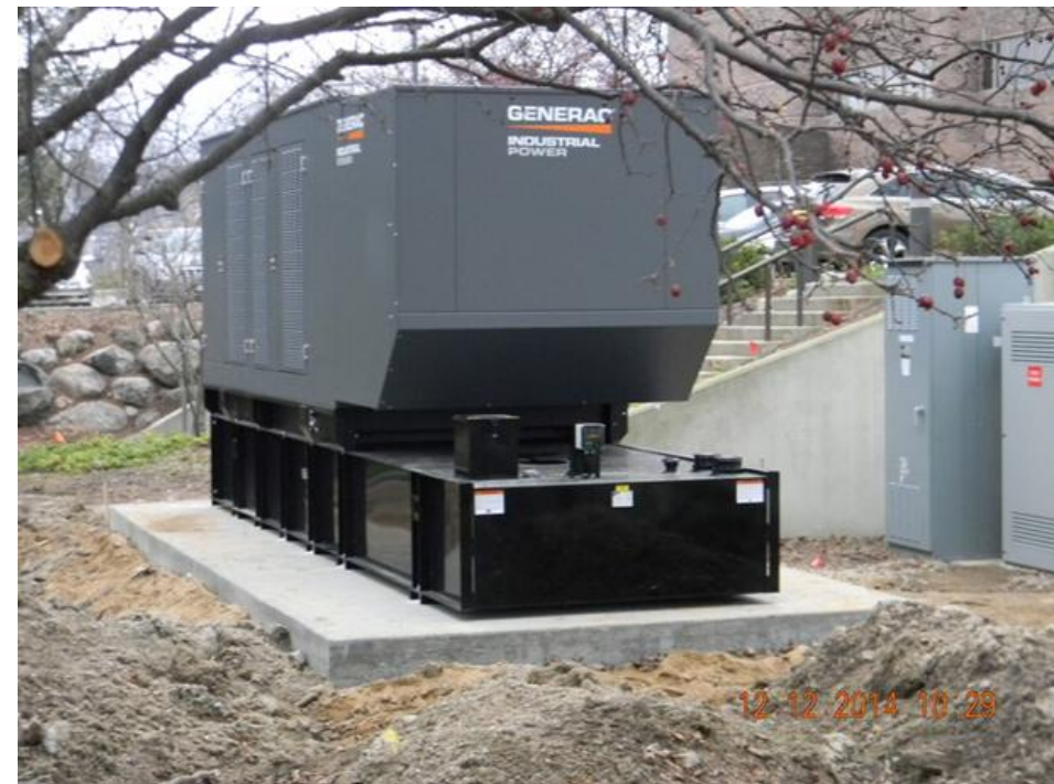
BUILDING WIDE BACK-UP GENERATOR
