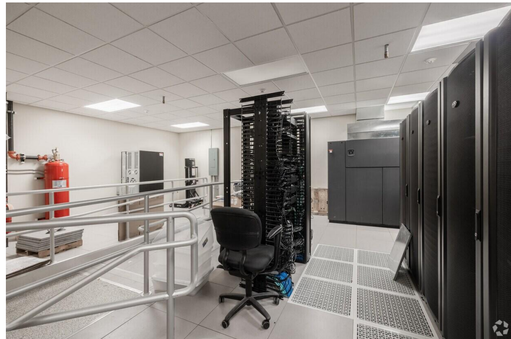
DEDICATED IT SERVER ROOM
