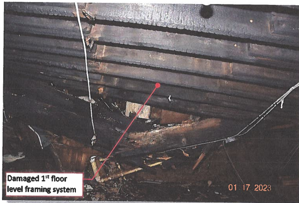
Pic. 23: View of the damaged first-floor level joist @ unit #1085
