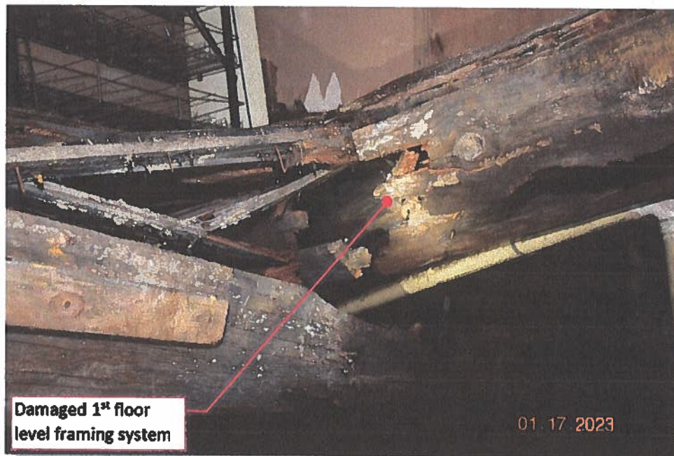
Pic. 22: View of the damaged first-floor level joist @ unit #1085
