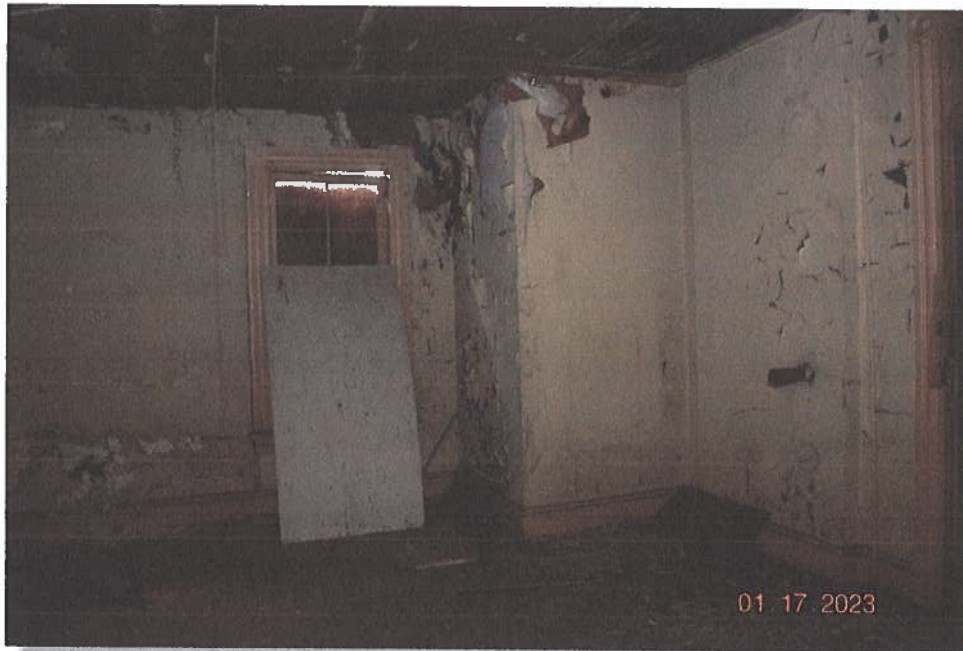
Pic. 26: Typical view of the cracks in the interior walls on the third-floor level
