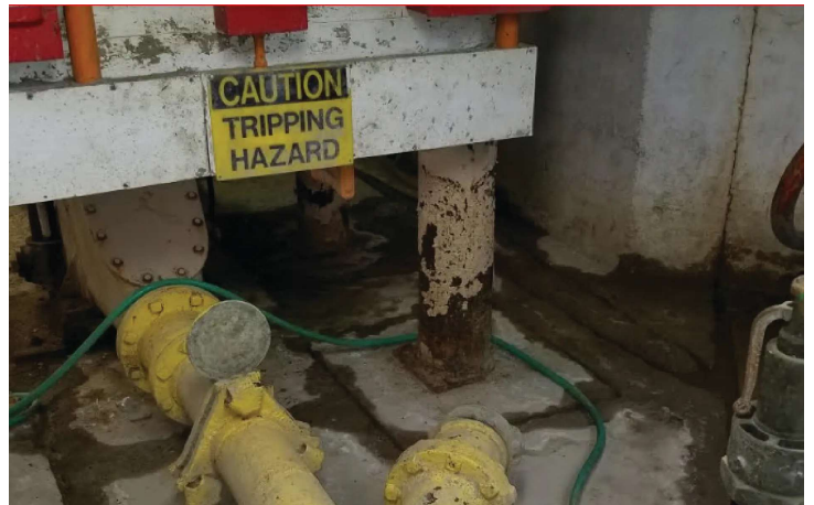
Basement FK Pump
