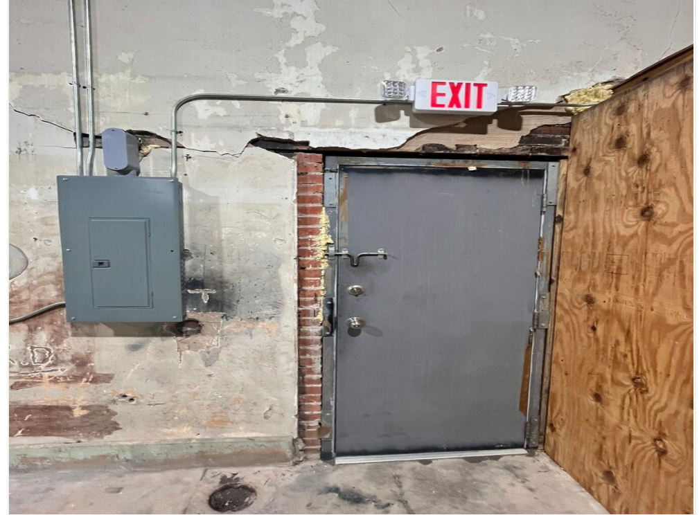
View of Brand New Breaker Box and Exit Signage
