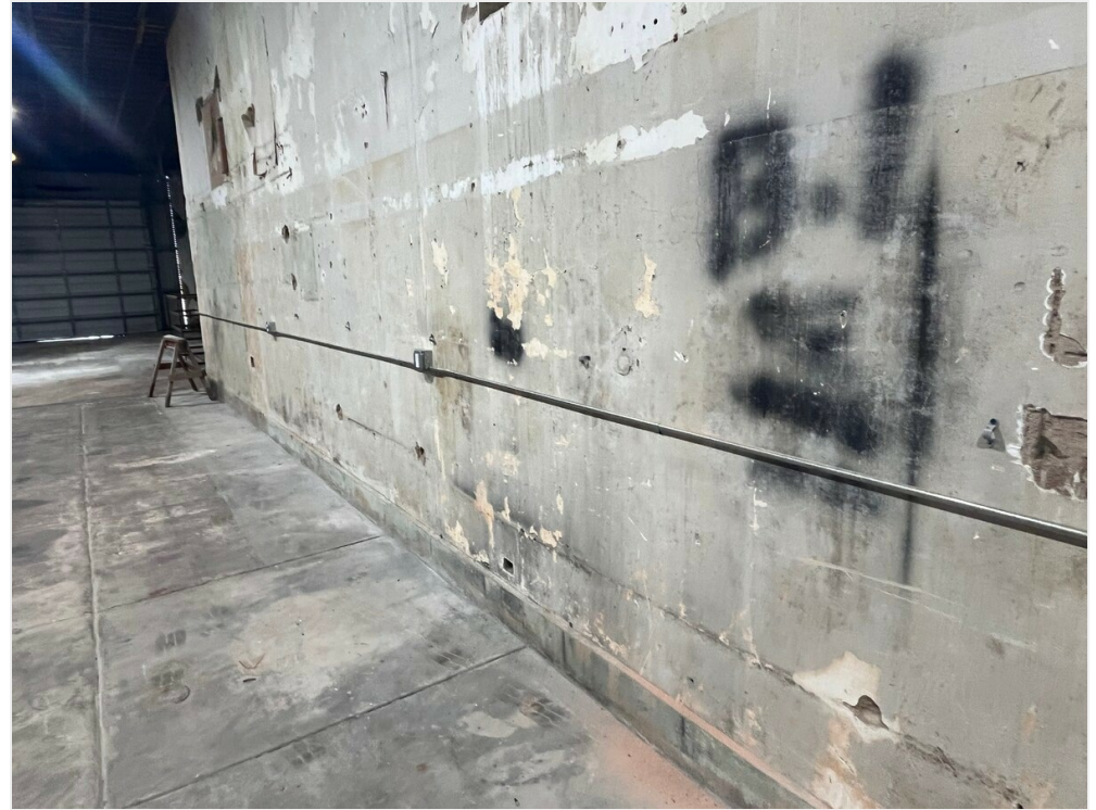
View of Brand New Electric (outlets, etc)
