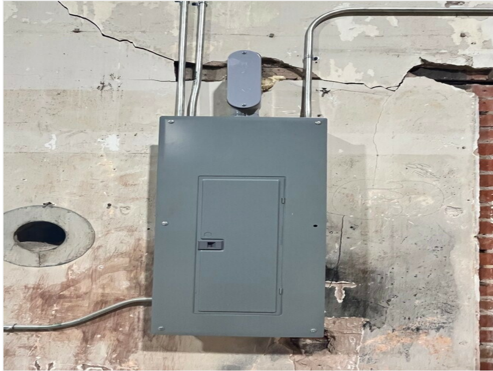
View of Brand New Breaker Box
