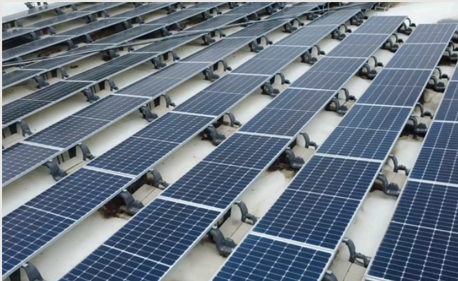
Large Solar Power System
