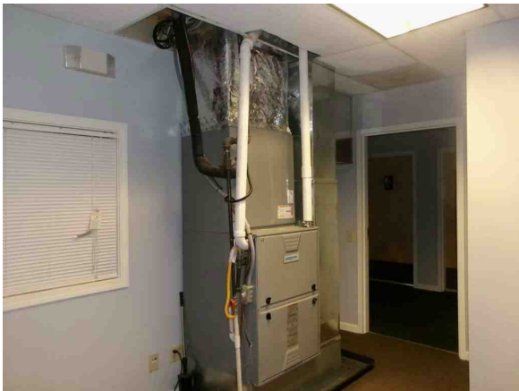
Level One HVAC
