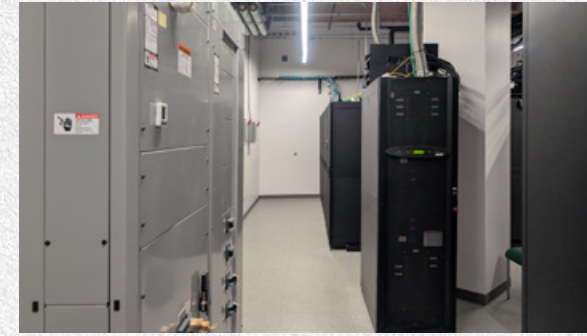
ELECTRIC CONTROL & SERVER ROOM
