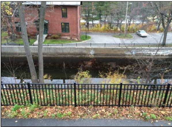
Photo 9: Canal wall showing presumed concrete patch (R) of penstock #1 which fed tailrace #1 until circa 1954 (EEM, 11/19/15).
