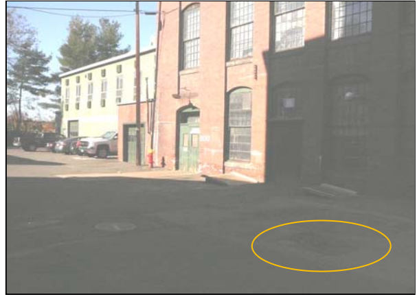
Photo 8: Catch Basin reported to drain into tailrace #1. (OHI, 11/16/15).
