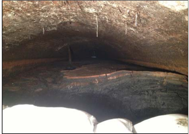
Photo 2: 7/9/15: 4 feet of material in tailrace described as gelatinous, saturated, unstable. Light at rear is reported to be from the CB between EEM buildings, other side of Bldg 28.
