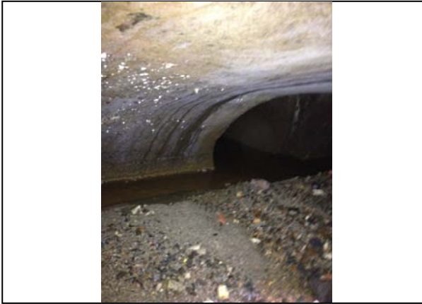
Photo 7: Material within the Flood Gate Chamber prior to clean out. (GZA/Gardner, 6/8/15).
