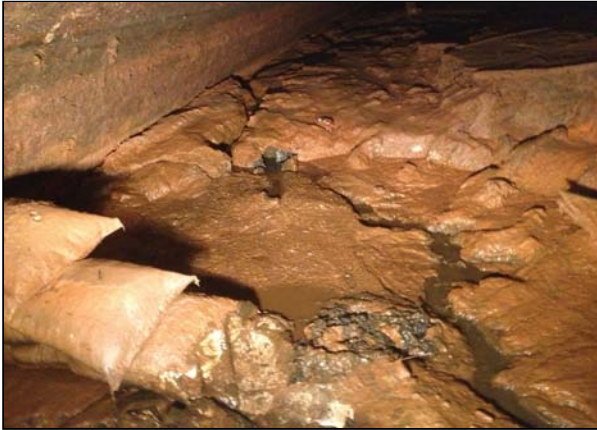
Photo 1: Sandbags breached by sloughing material. "tailrace" sample collected rear center. 9/28/15
