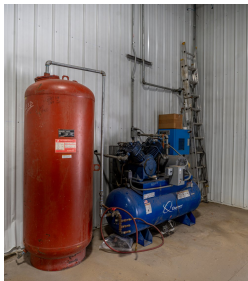
15 HP air compressor
