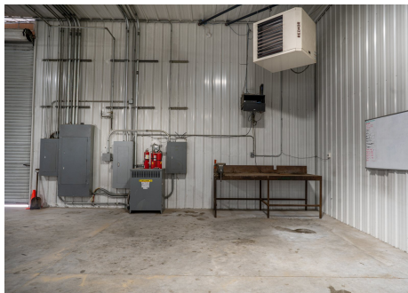
800A three-phase service & transformer
