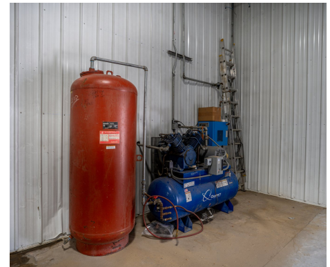
15 HP air compressor in place
