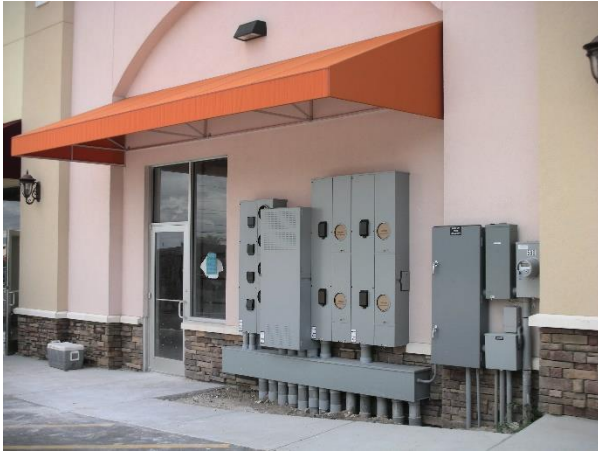
Not Allowed (utilities facing street)
