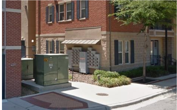
Not Allowed (not facing the street, but still visible)
