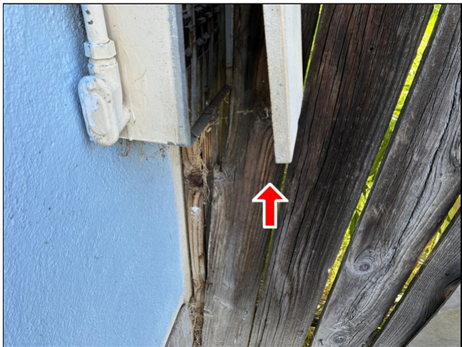
6.1 Item 3(Picture) Stuck panel cover
