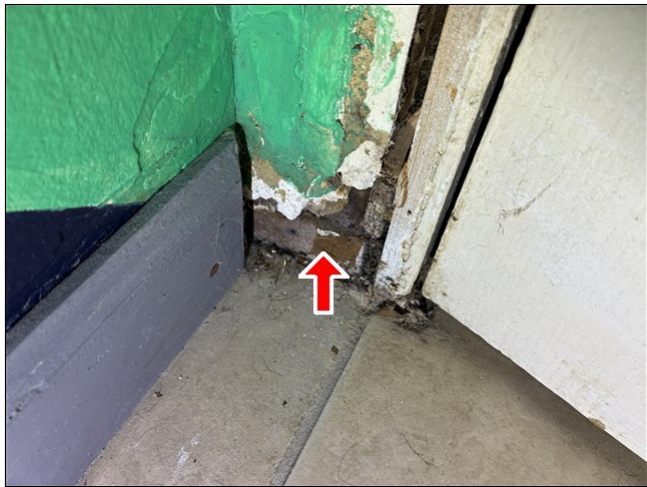
10.1 Item 1(Picture) Behind bathroom door
