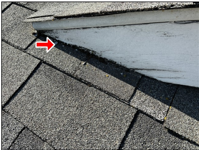
3.6 Item 9(Picture) Barge board touching roof
