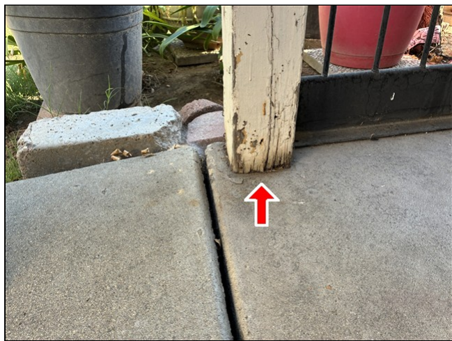
3.9 Item 1(Picture) Wood-cement contact may wick moisture, damaging wood
