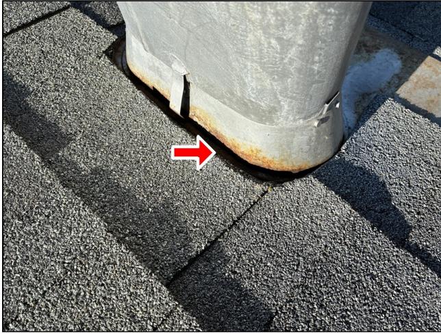
4.2 Item 3(Picture) Rusted vent penetrations
