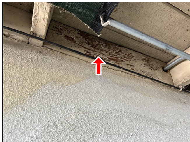
3.3 Item 3(Picture) Eaves paint peeling
