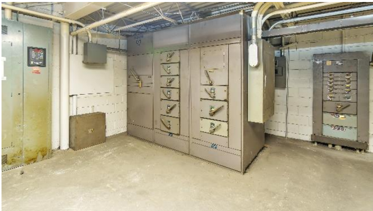
Heavy Electrical Service – 2000 amps
