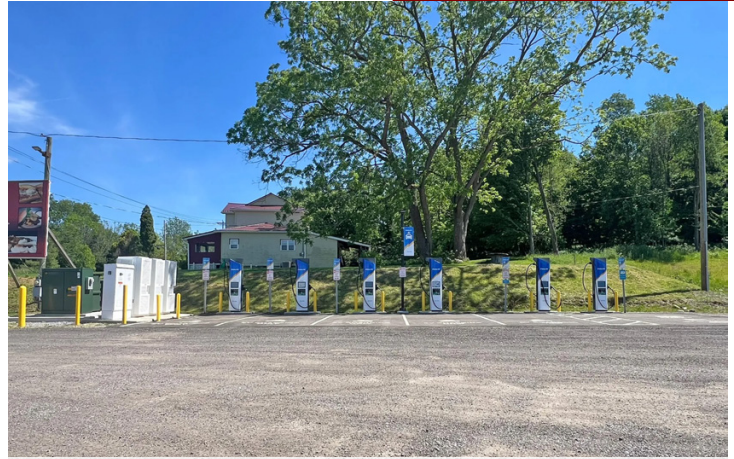
EV Charging Stations On-Site
