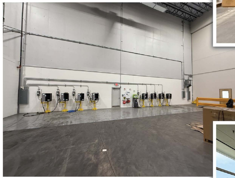
Forklift Charging Stations
