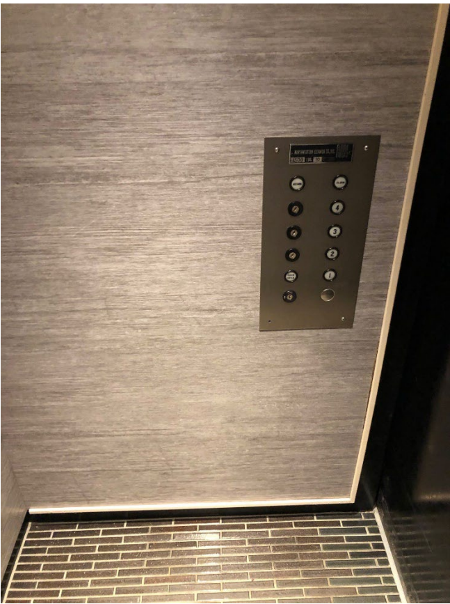
Simple, smartly finished elevator cab
