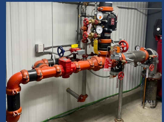
Newly Upgraded Sprinklers
