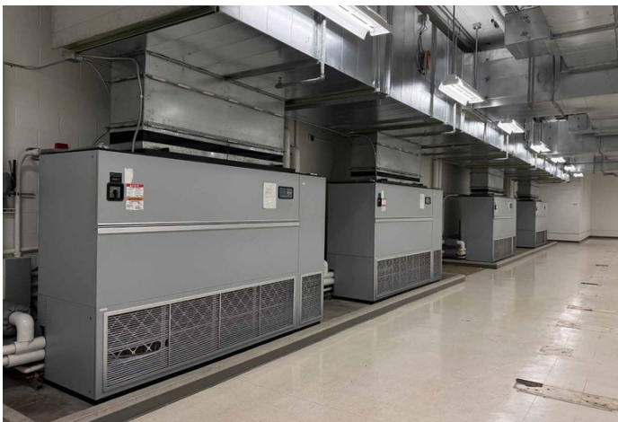
Existing cooling equipment.
