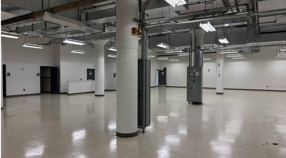
Open lower-level space and electrical infrastructure.
