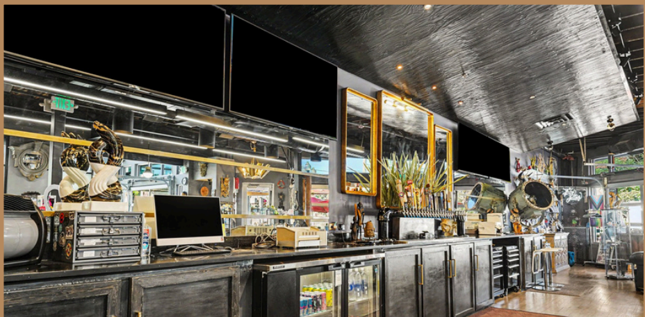
The back bar area, including tap tower, refrigerators, bar canopy, and plumbing remain in place.
