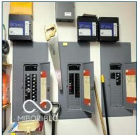
Mechanical room electrical box
