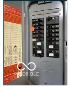
Electrical box in pantry
