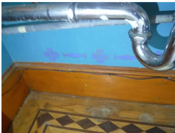
31. Item 2N Interior plumbing leaks/stains (Chalet)
