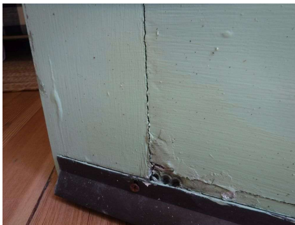
7. Item 1L Damaged Manzanita cottage wood sample
