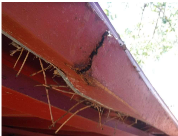
1. Item 1A Damaged & leaking gutters sample
