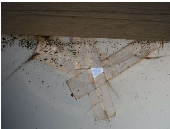
25. Item 2E Cracked skylight at barn house
