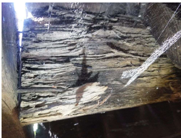
5. Item 1J Damaged decks framing & wood sample #2
