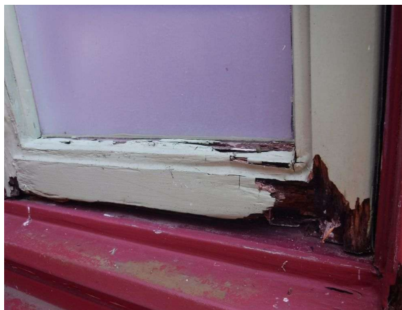
14. Item 1P Damaged Oak Hill cottage wood sample #2
