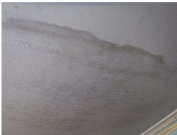
35. Item 4E Moisture stains on basement ceiling sample
