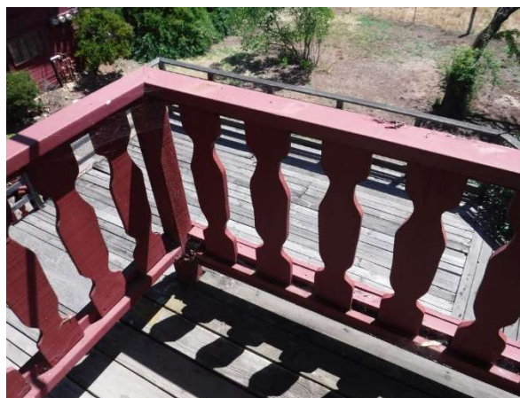
6. Item 1J Damaged main house decks safety hazard sample
