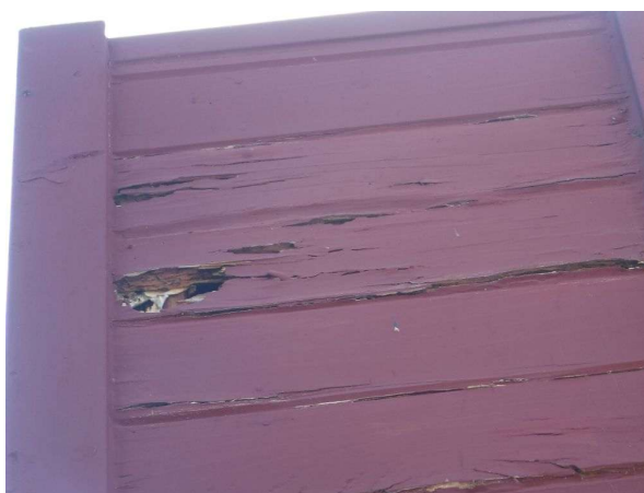
15. Item 1P Damaged Oak Hill cottage wood sample #3
