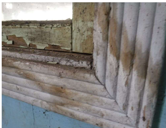
36. Item 4H Moisture stains basement window trim sample
