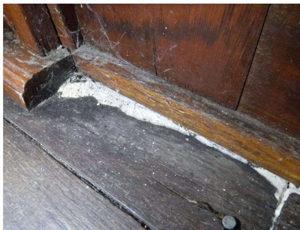
26. Item 1I Moisture stains/fungus at wood door areas
