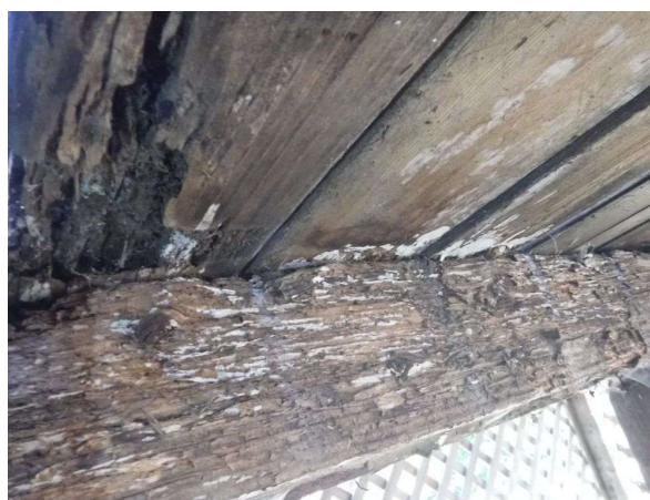
4. Item 1J Damaged decks framing & wood sample
