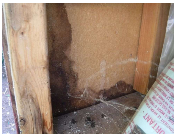
10. Item 1L Damaged Manzanita cottage wood sample #4
