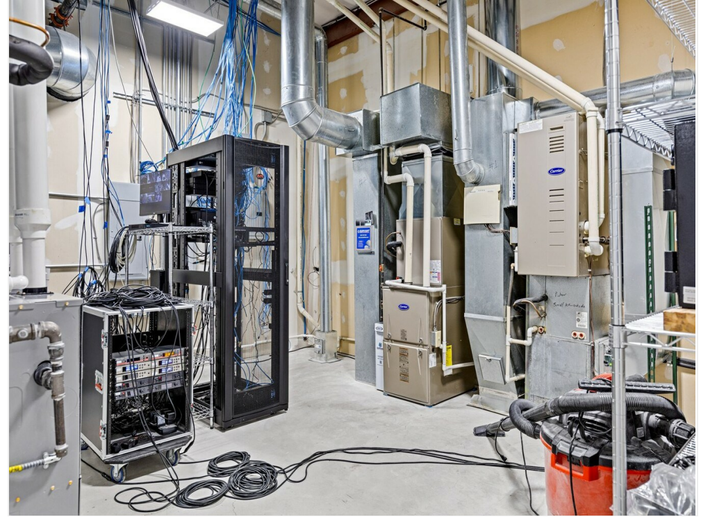
2nd Floor HVAC
