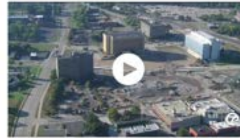
An aerial view shows the remaining, six-story structure of the Phoenix Center with its demolition. The project was owned by Phoenix Center Development LLC.
