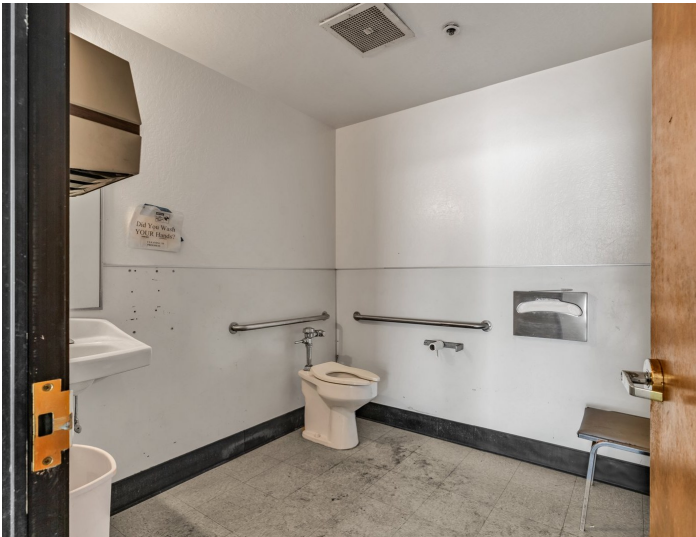
On-site ADA-compliant restroom
