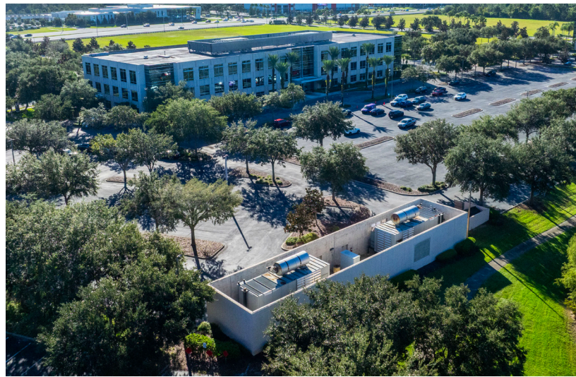
REDUNDANT POWER BACKUP TWO GENERATORS IN PLACE
