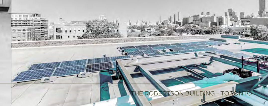
Solar Power Panels
