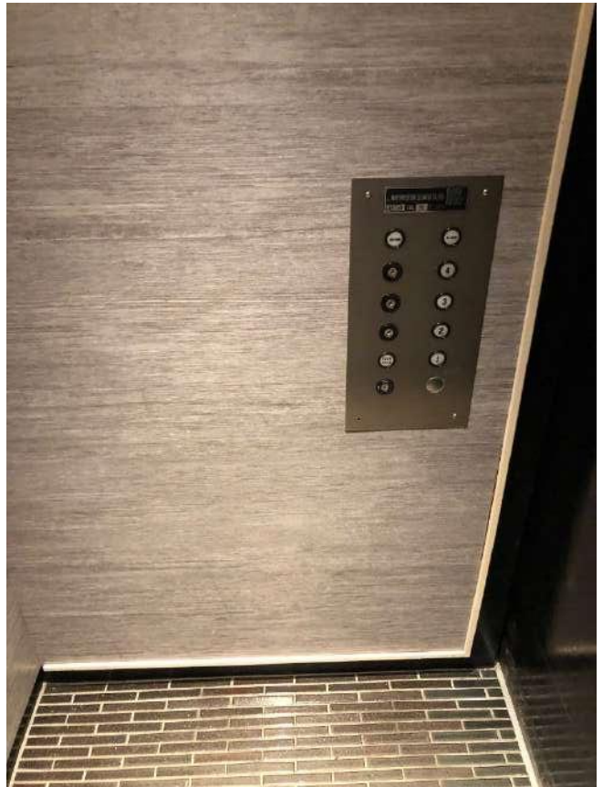
Simple, smartly finished elevator cab
