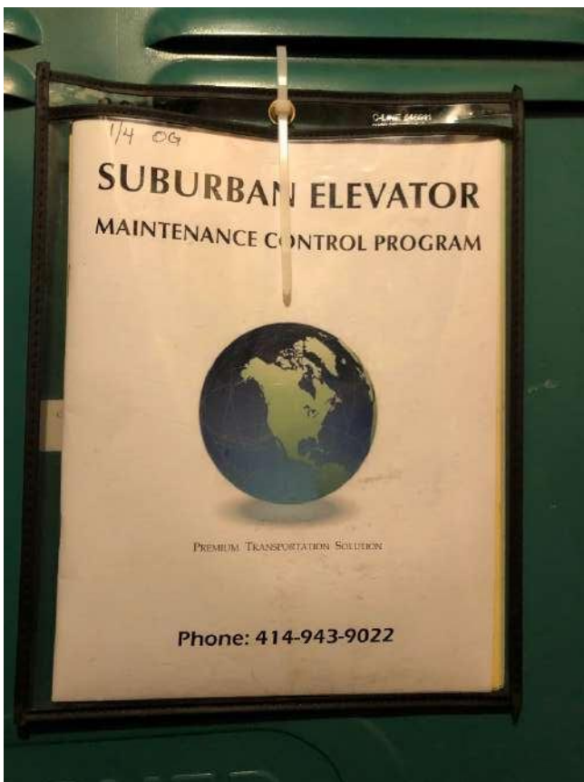
Properly maintained hydraulic elevator
