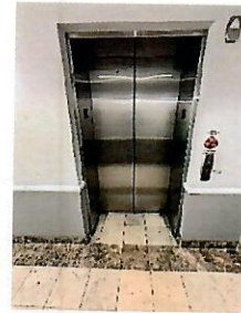
OTIS 3,000 lb. capacity elevator
