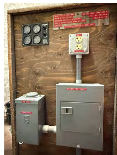
Control panel for 8kW Northern Lights diesel backup genset
