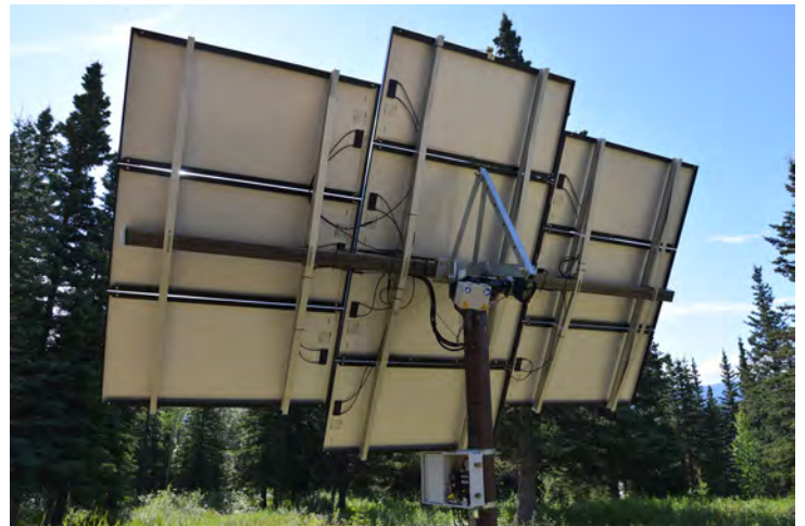
Series wiring of 2 panels for 85.4v to charge controller and 48v battery bank
