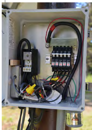
Array junction box, 10 modules w/2 each wired in series on a DC breaker
