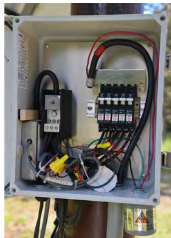
Array junction box, 10 modules w/2 wired in series on a DC breaker
