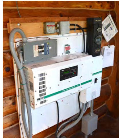
Trace/Xantrex SW5548 inverter/charger & Outback controller
