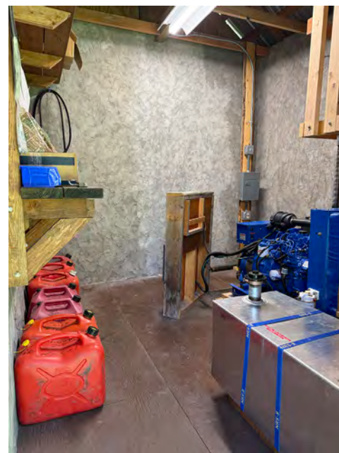
Inside Generator Bldg, 8kW genset
