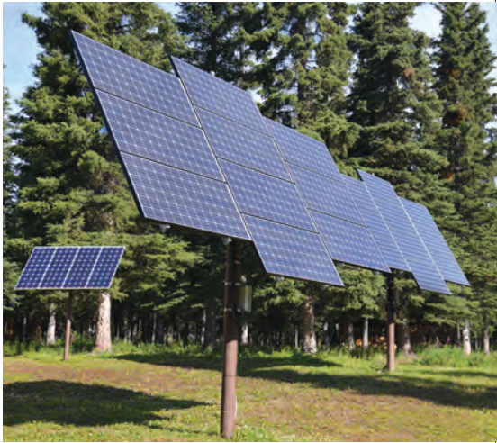
4.4 kW azimuth tracking arrays
