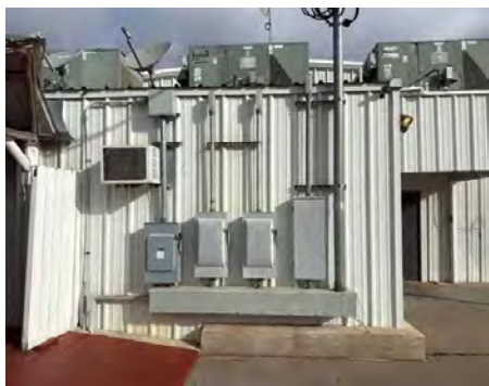
Rear: Main Disconnects
