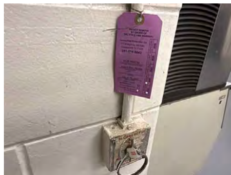
Fire Suppression System
