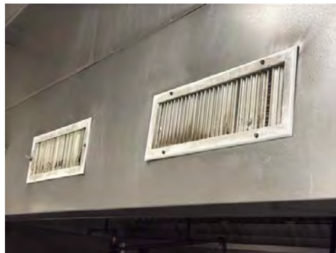
Make up Air dirty
