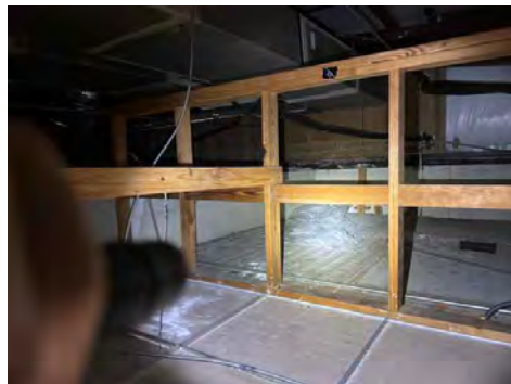
Above walk-in coolers
