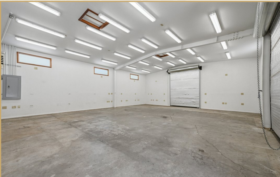
Renovated Shop — 400A 3-Phase
