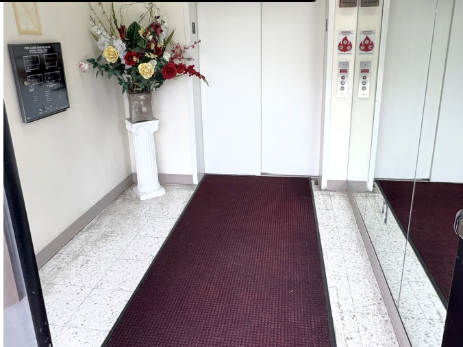
Elevator | ADA Accessibility
