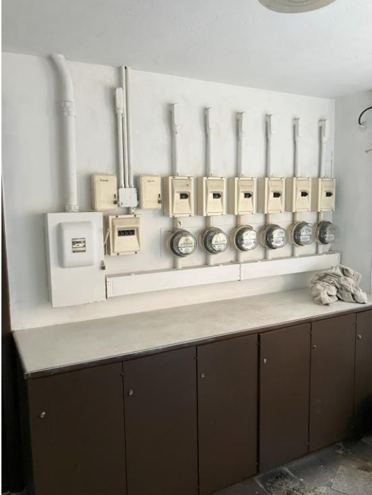
Typical electrical meter area of laundry rooms
