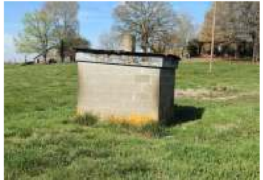
14) A water supply well observed on the central portion of the site.
