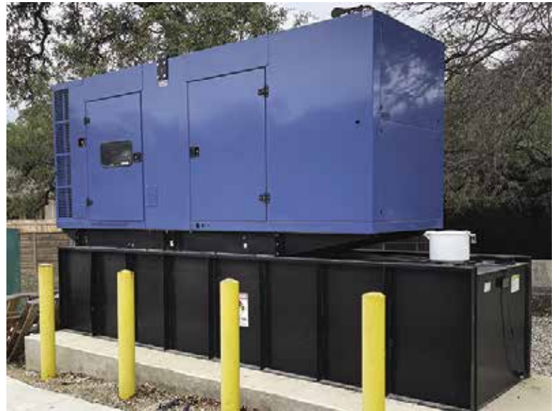
500 KVA BACKUP GENERATOR
