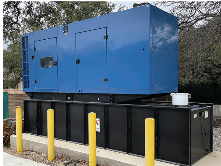
500 KVA BACKUP GENERATOR
