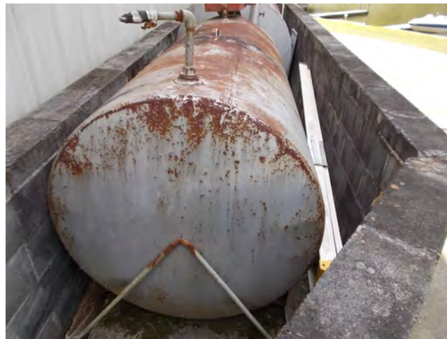
500 gallon AST and retaining wall surrounding tanks.
