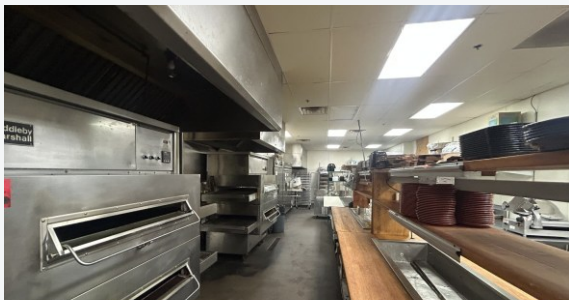
Commercial exhaust hood and cook line
