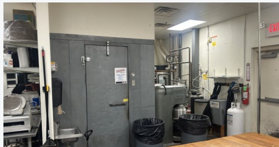
Walk-in cooler and back-of-house
