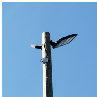
LED POLE YARD LIGHTING
