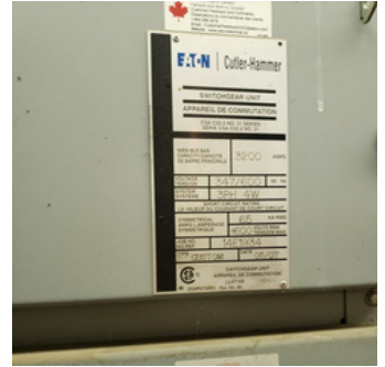
3-PHASE 3,200 AMPS / 500 VOLTS
