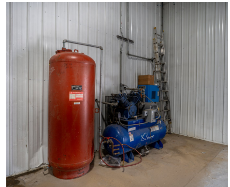
15 HP air compressor (Unit B)
