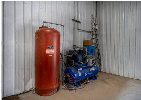
15 HP air compressor (Unit B)
