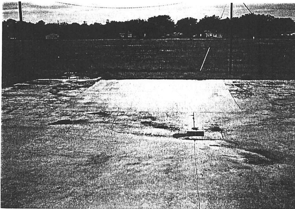
View of abandoned underground storage tank area -- note newer concrete near grass
