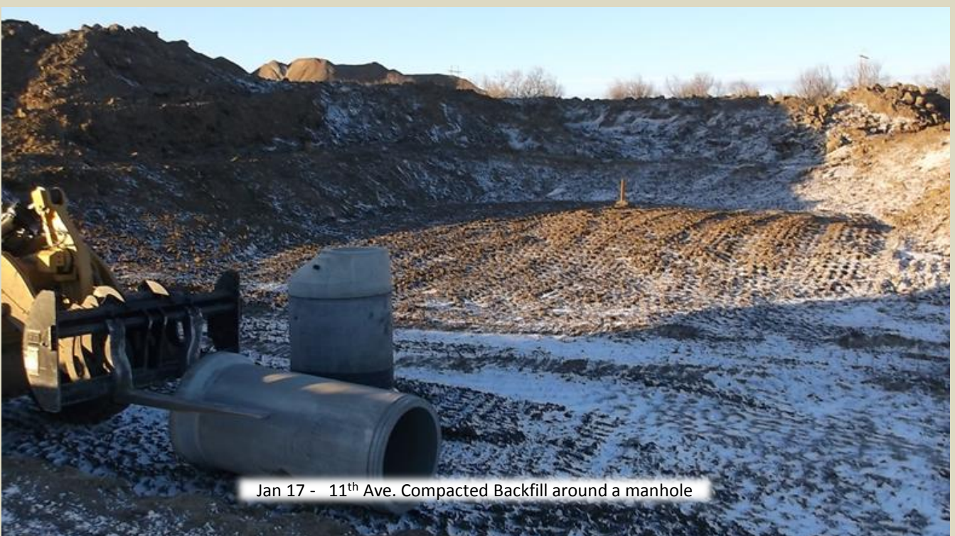
Jan 15 - 11 th Ave. Storm Crew installing 36" RCP South from one of the manholes
