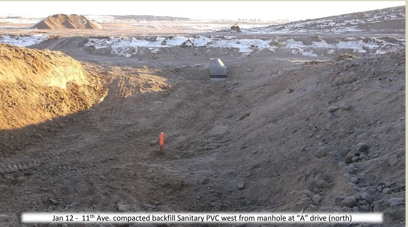
Jan 12 - 11 th Ave. Sanitary Crew Trenching for PVC run west down "A" drive (south), and "B" drive
